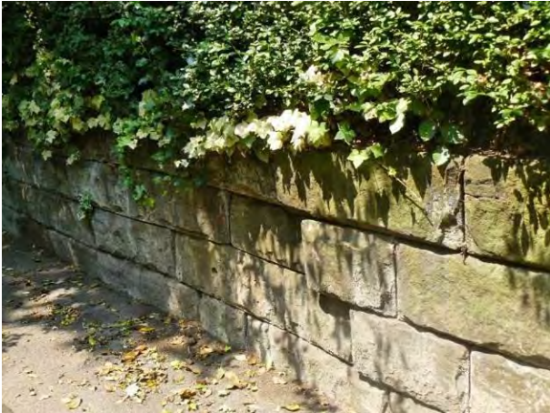
Damaged wall on Harrop Road
