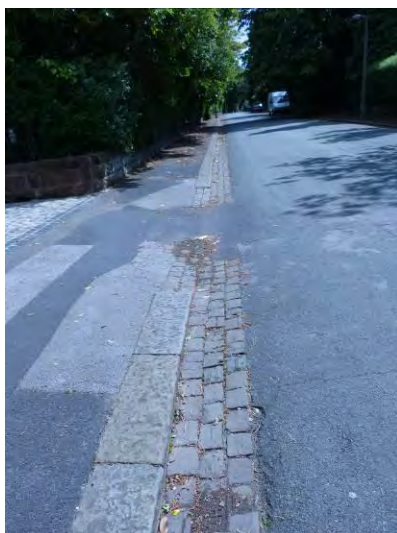
An example of cobbled setts, historic kerbstones and ad hoc tarmac repairs, as well as a good example of modern setts to the driveway.
